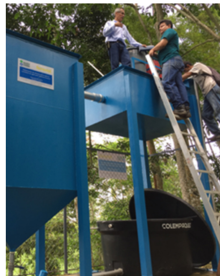
Lisboa Water treatment plant built by the Ruta del Cacao project.
